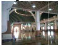
Figure 32. Purlins form a brilliant geometric pattern on the ceiling. Masjid Agung, Central Java.
